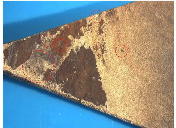
Figure 3. Section of pipework with pitting revealed after partial removal of surface deposits.
