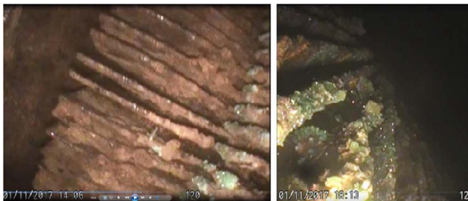
Figure 2. Internal inspection pictures of cooler/condensers' heat exchanger surfaces.
