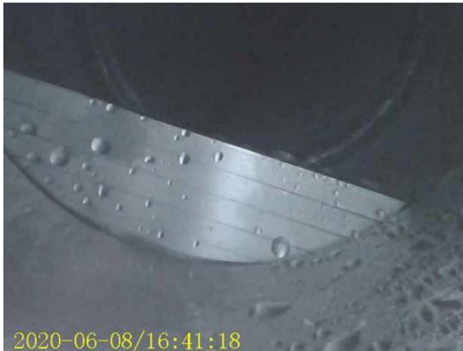
Figure 25. Condenser outlet camera showing the dam installed for Dryer 3. Water droplets and a pool forming can be seen during regeneration on 8 June 2020.
