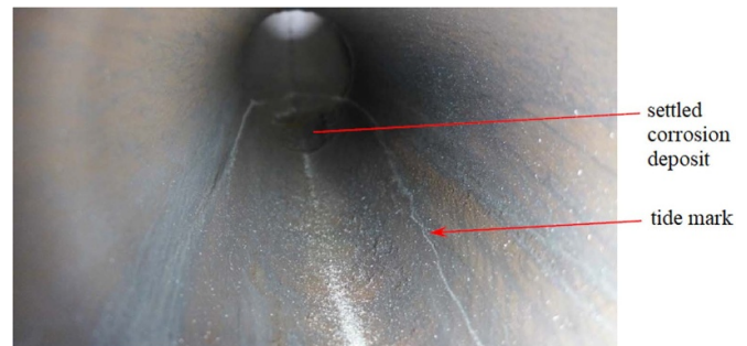
Figure 4. Internal image of 5 inch pipe demonstrating settled deposits and the presence of a tide mark.
