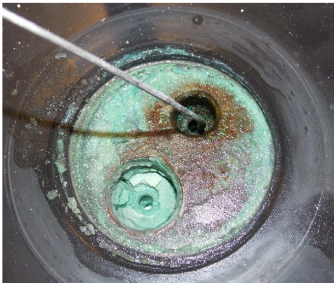
Figure 15. Corrosion product build-up on bottom flange and inlet pipework during acute HF testing Intersorb (note larger penetration was not used).
