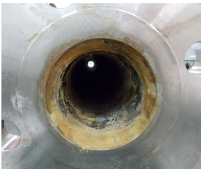
Figure 16. Corrosion within the inlet of the test rig column during acute HF testing Intersorb.
