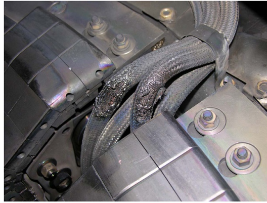
Figure 12. C-Mod SXR signal cables damaged by a RE strike. Several cubic centimeters of steel, copper, Teflon, and fiberglass were blasted out of the SXR signal cables.
