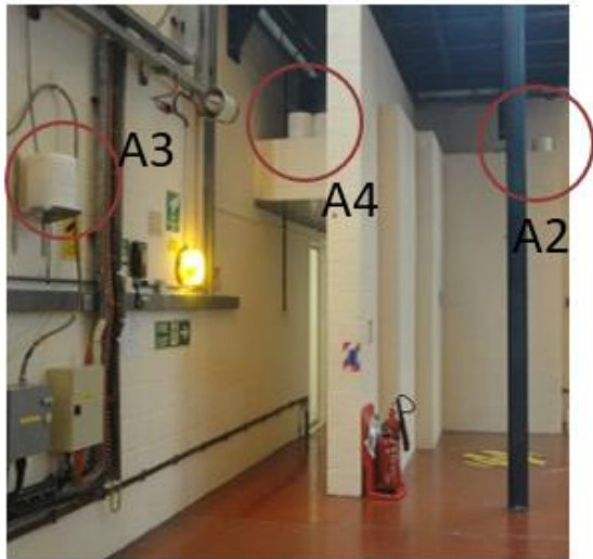
Figure 3. A2, A3 and A4 experimental location circled with red photographed during installation.
