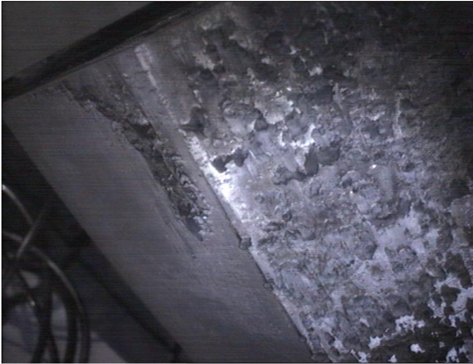
Figure 45: View of part of the apron of a Tile 1 (right-hand side) and the upper front face of the tile (towards the left-hand side) during the 2007 JET shutdown inspection, showing spalling deposits. The tile had been exposed 1998-2007.
