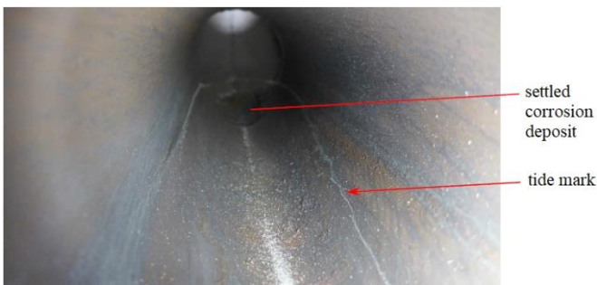
Figure 3 – Internal image of 5" pipe demonstrating settled deposits and the presence of a tide mark
