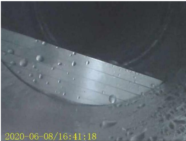
Figure 24 - Condenser outlet camera showing the dam installed for Dryer 3. Water droplets and a pool forming can be seen during regeneration on 8th June 2020
