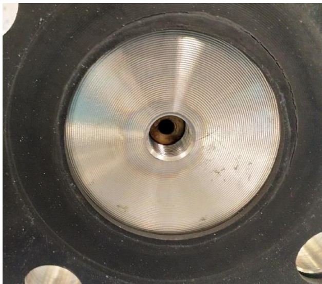
Figure 16 - light pitting corrosion on outlet flange during acute HF testing Intersorb
