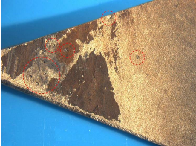
Figure 2 – Section of pipework with pitting revealed after partial removal of surface deposits
