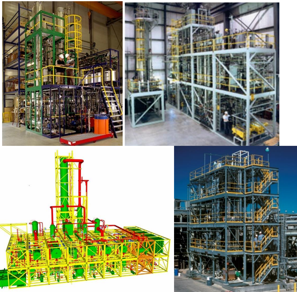
Figure 2 - Factory-built process plant modules (Bramsiepe et al., 2012) by ((Zeton, 2021))
