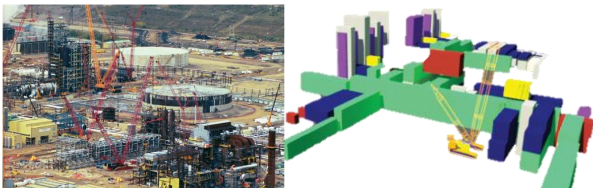
Figure 11 - Optimised crane planning and configuration for a modular project in Alberta, Canada (Taghaddos et al., 2018)
