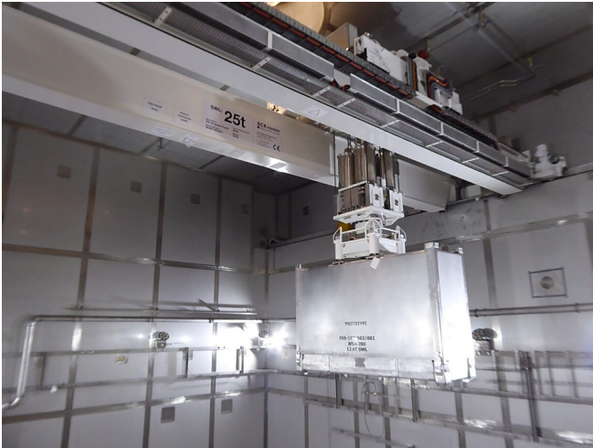
Fig. 10. Grapple crane carrying stainless steel waste storage basket.
