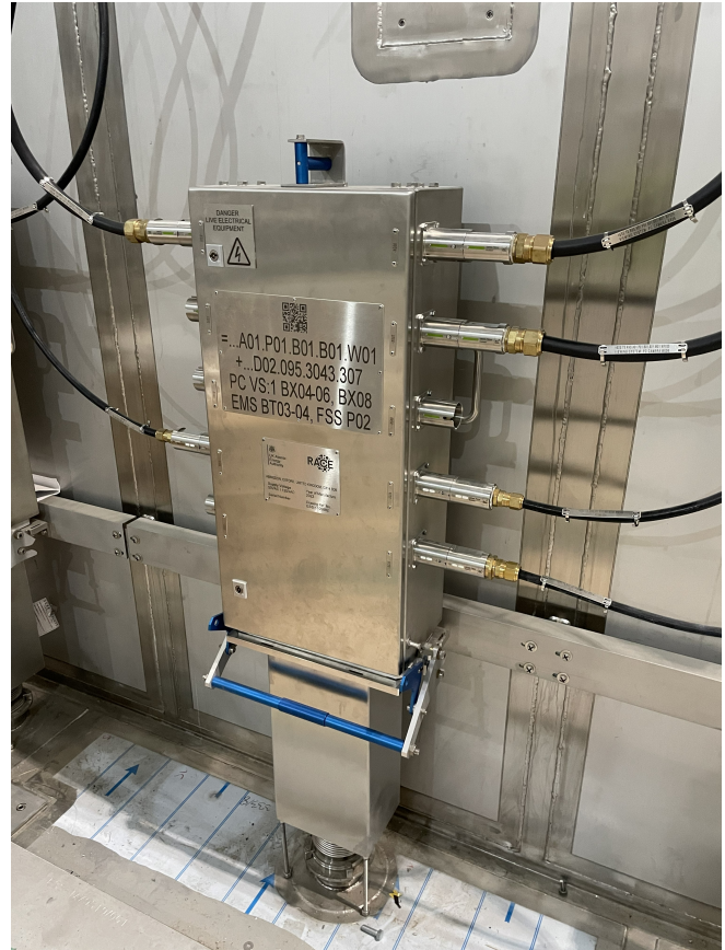
Fig. 3. Electrical Junction Boxes installed within the Active Cells Facility.
